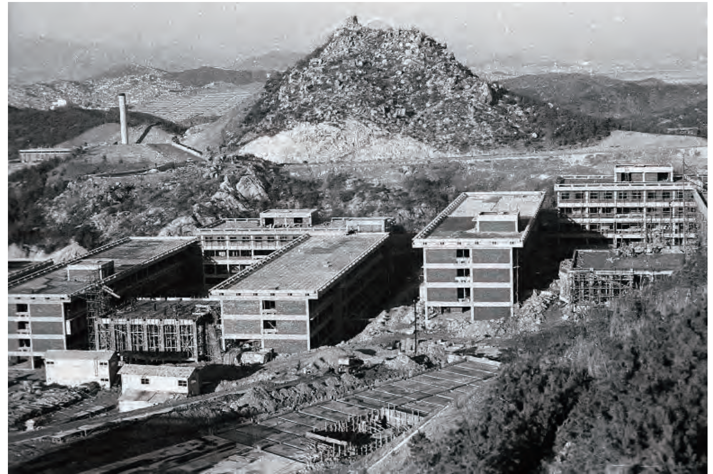
1975.1.1. 5-12동 (인문관, 사회과학관, 사범관) 건설 현장 Buildings 5 to 12 (Humanities, Social Sciences, and Education) under construction
